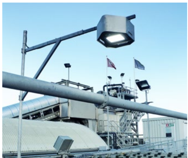
Metris addIQ RheoScan installed at a belt filter press
